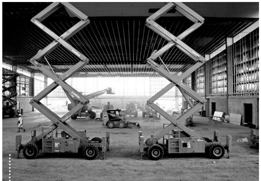
Work on the 3,705 square metre Sports Stadium, which will be used for University and community sporting events and USC ceremonies, began in November 2006.
