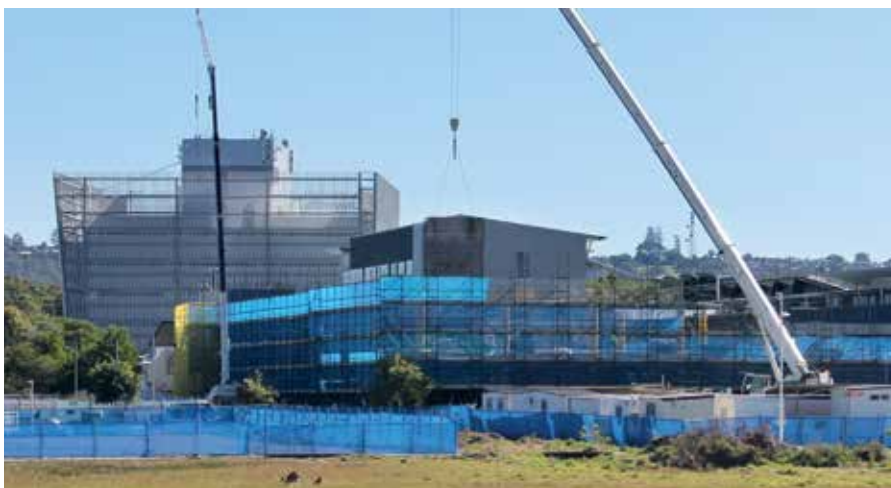
■ USC's Engineering Learning Hub is being constructed around two existing buildings (Buildings H and H1), with work due to be completed in early 2015.
